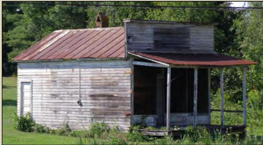
Store, Roanoke, VA (c. 1900) This example features a false front. (photo from DHR)
